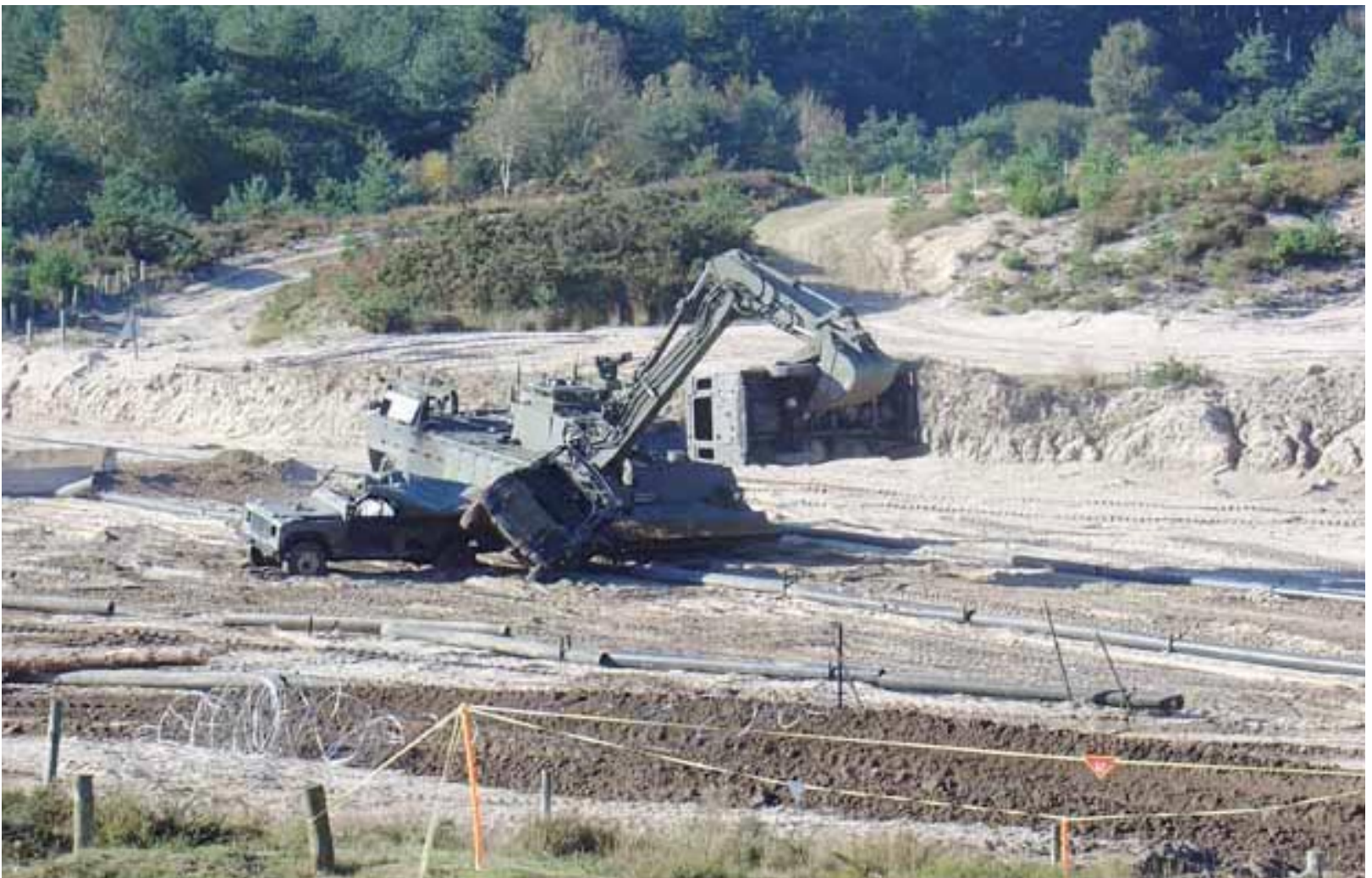
The need to clear barricades has increased in significance during recent urban operations. Here Trojan demonstrates that capability.
